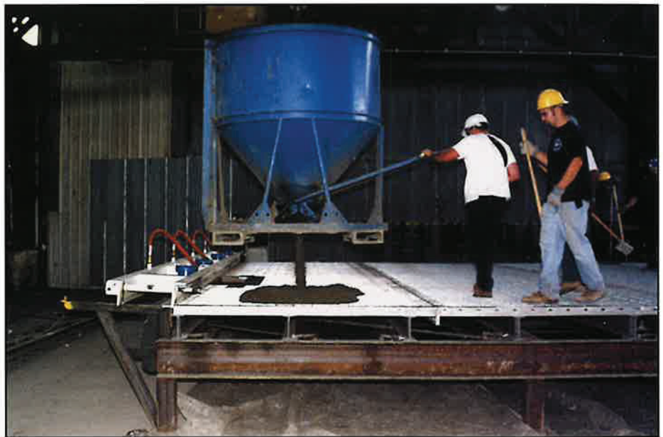
AC Miller Company precast grid units, using lightweight concrete, in their Spring City, PA facility.
