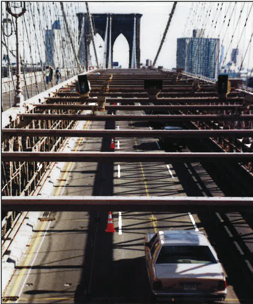
One of three traffic lanes available to contractor during limited daylight hours for preliminary saw-cutting.
