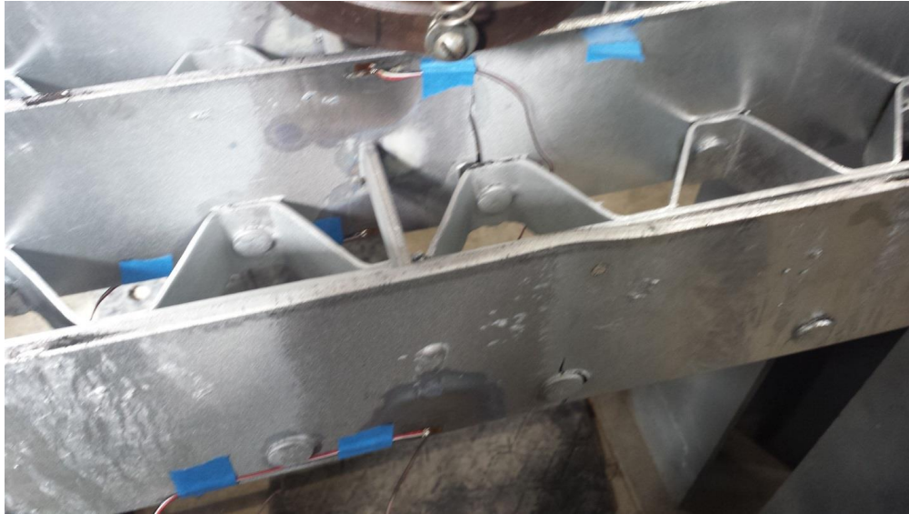
Figure 5.11 – 37R5 Lite Small Panel with fatigue cracks
